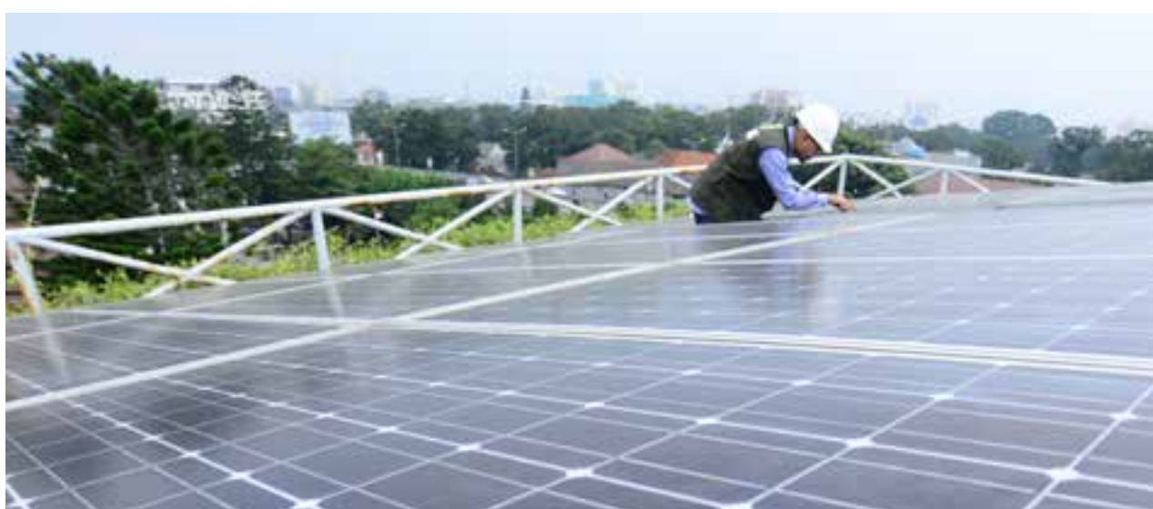
Bio Farma technician is maintenance on the solar cell to utilize the sun's energy as a natural electricity generator.
